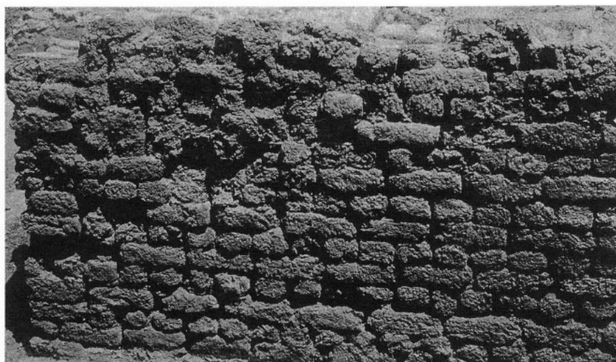
e. M. Q. T. Temple III-a, room (9), east wall, southern part, brickwork, looking down to east.
